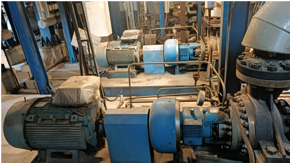
Figure 4. Circulation Pumps After Revision (360 t/h)
