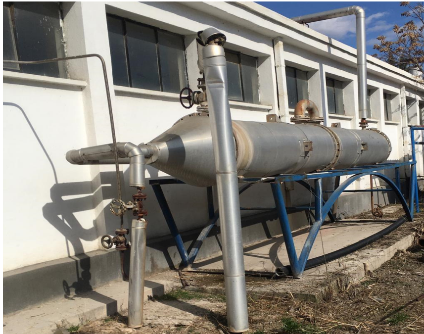
Figure 2: 2 st Stage Studies for Space Heating with Deaerator Exit Steam from Waste Steam in Ammonia Nitrate Production
